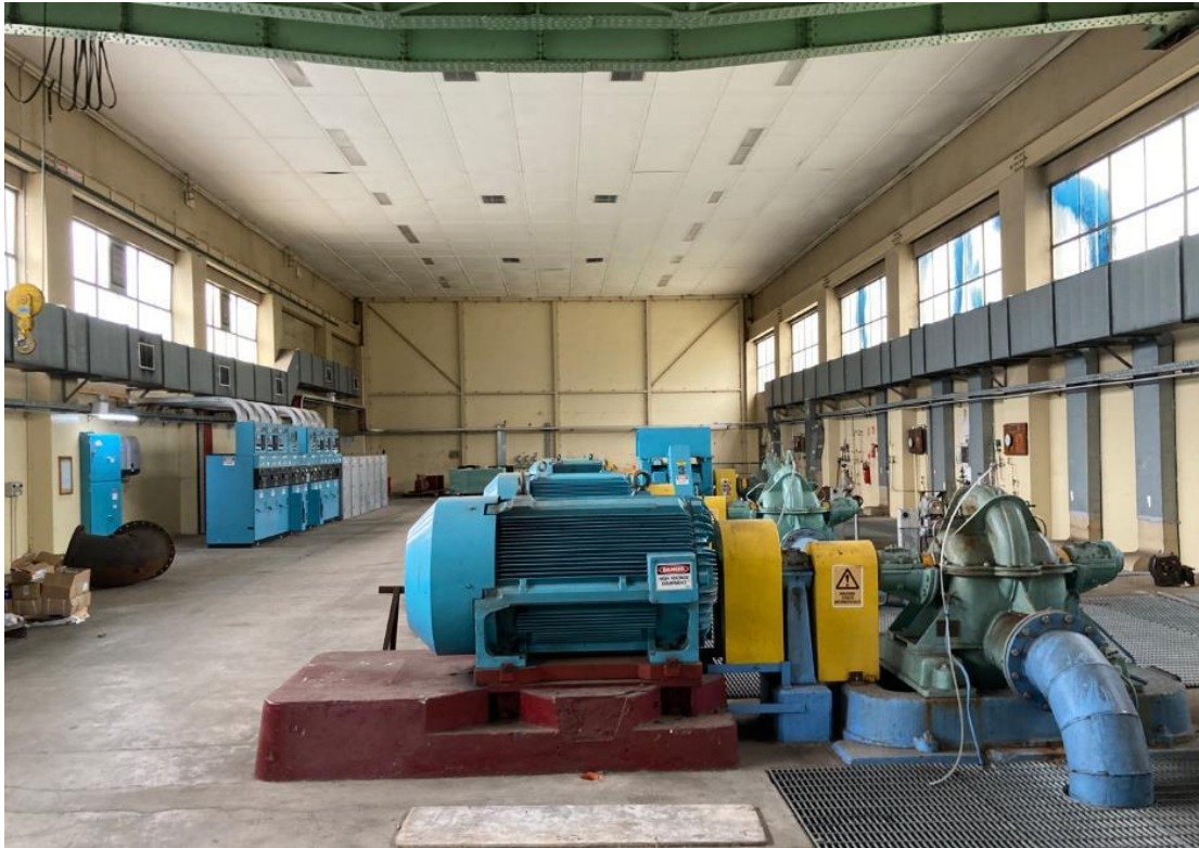
Figure 11: Internal view: Pump House
